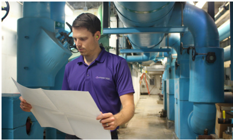
MECHANICAL, ELECTRICAL, PLUMBING
