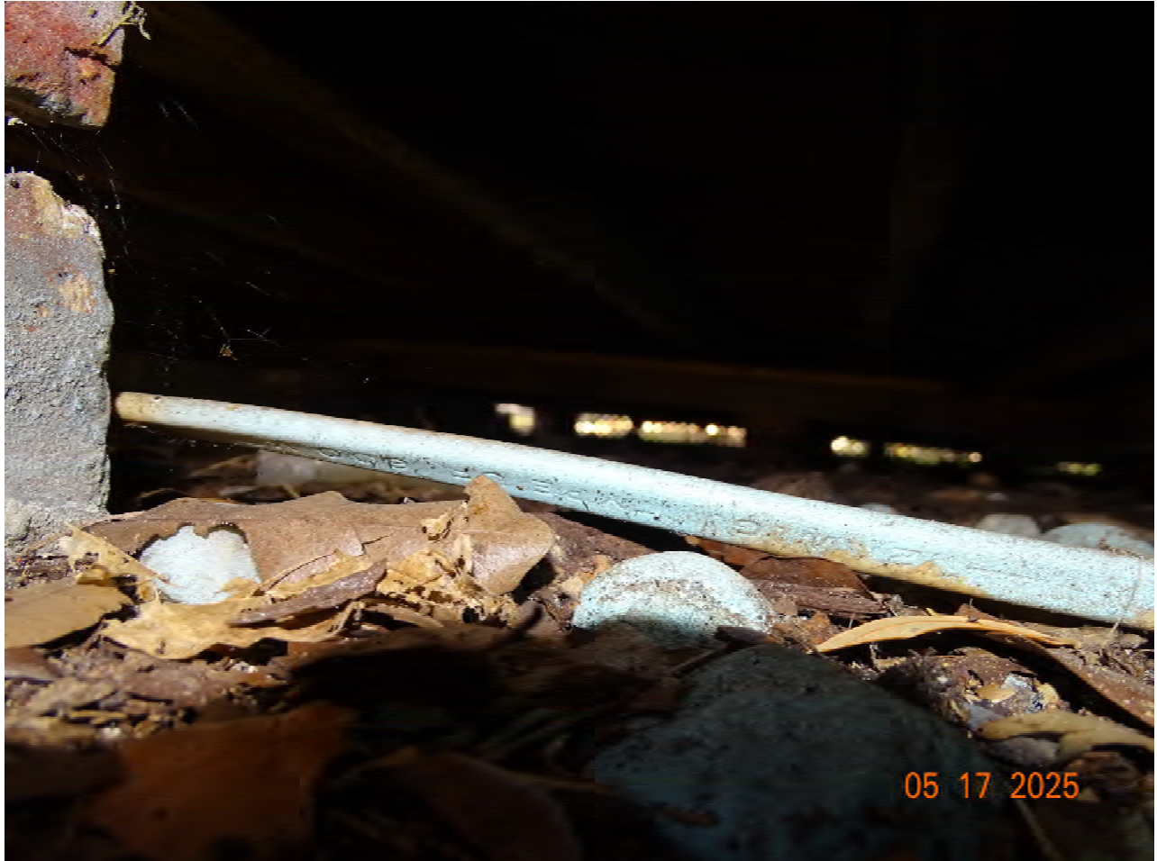
33 Displaced brick pier
