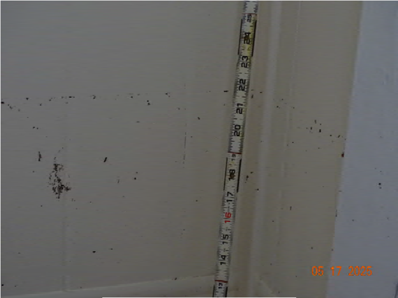
15 Water line inside
