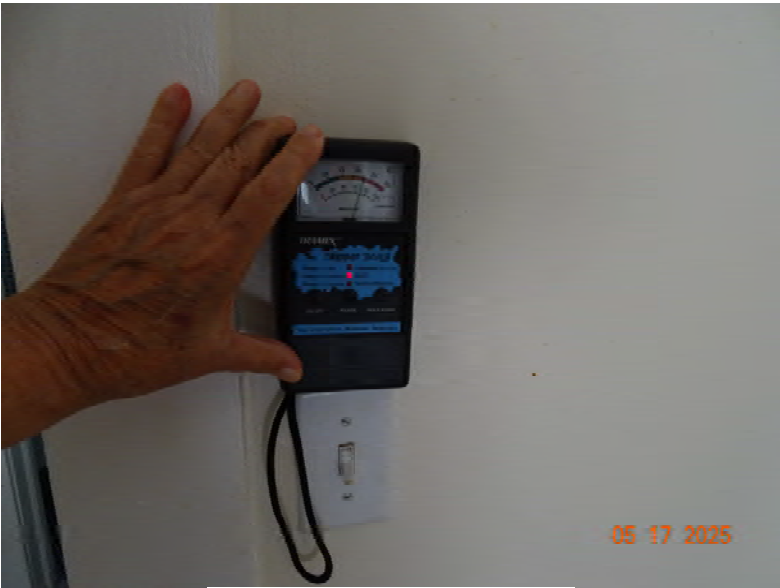
27 Moisture at wall
