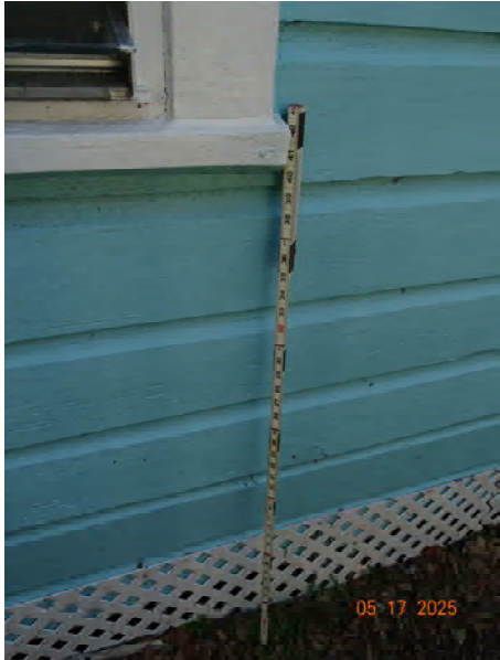
08 Water line 40 inches above gro
