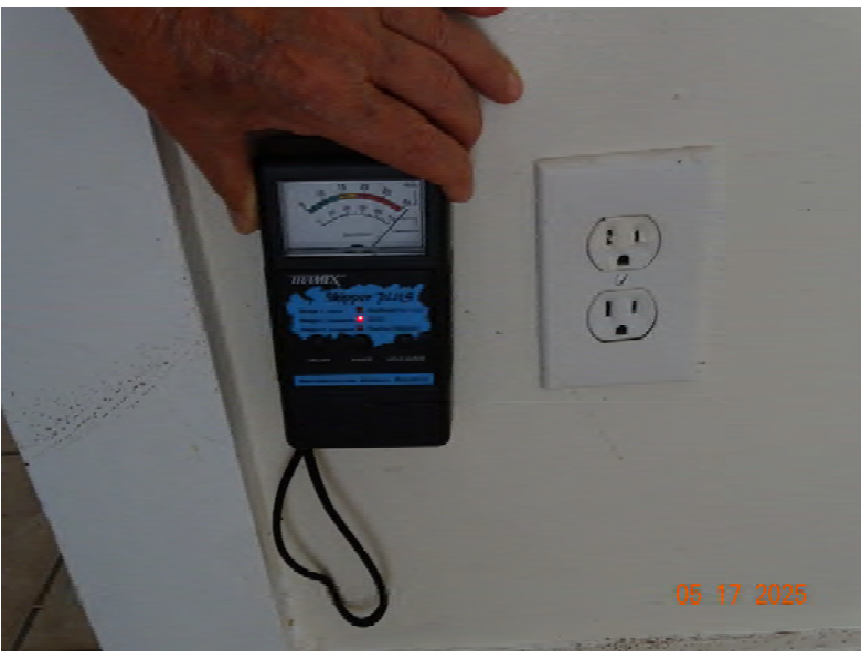
25 moisture at wall
