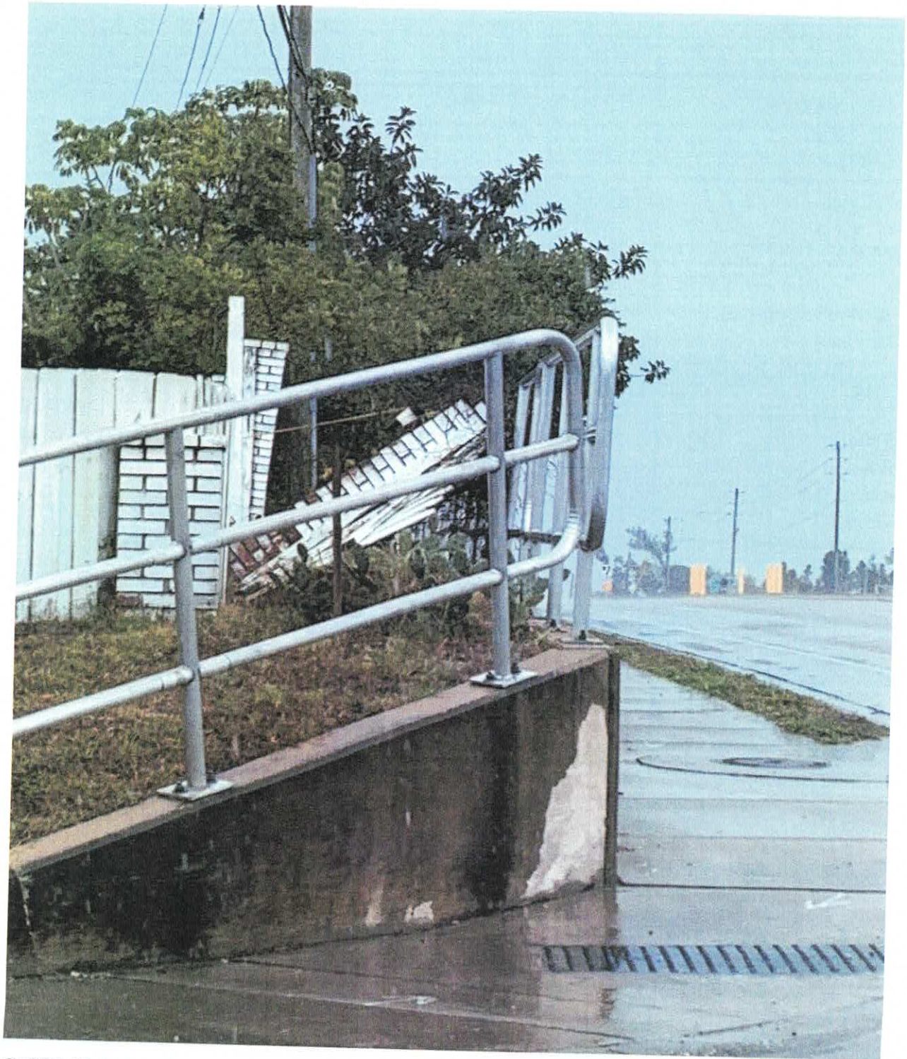
CASE # 25-80000431 SITE: 300 LEAFWOOD RD TARPON SPRINGS, FL 34689 INITIAL INSPECTION: 2/25/2025 BY CEO MROLLESTON
