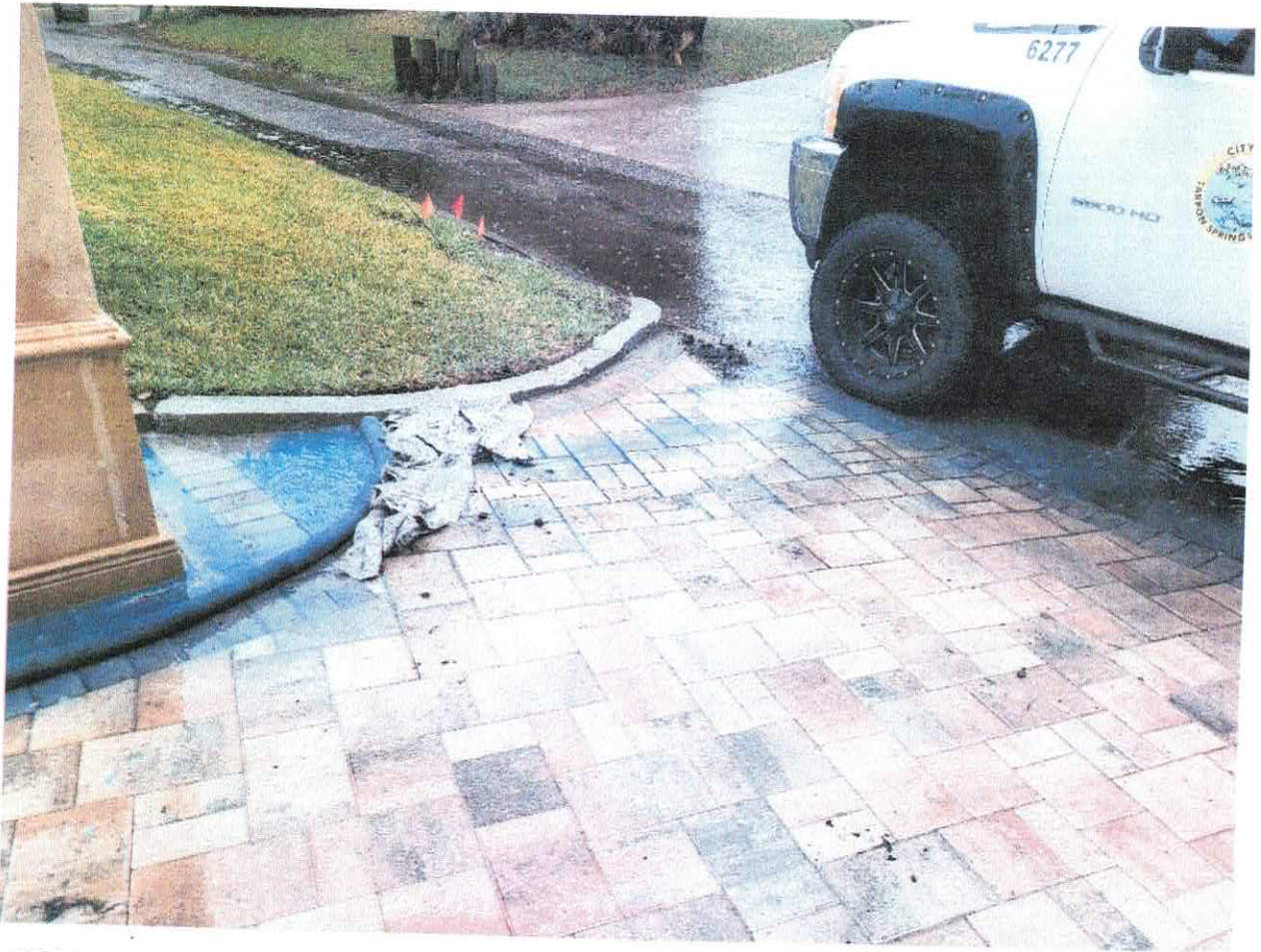
CASE 25-80000428 SITE: 1403 CIRCLE DR INITIAL INSPECTION 2/20/2025 STORMWATER - PAUL HOPKINS
