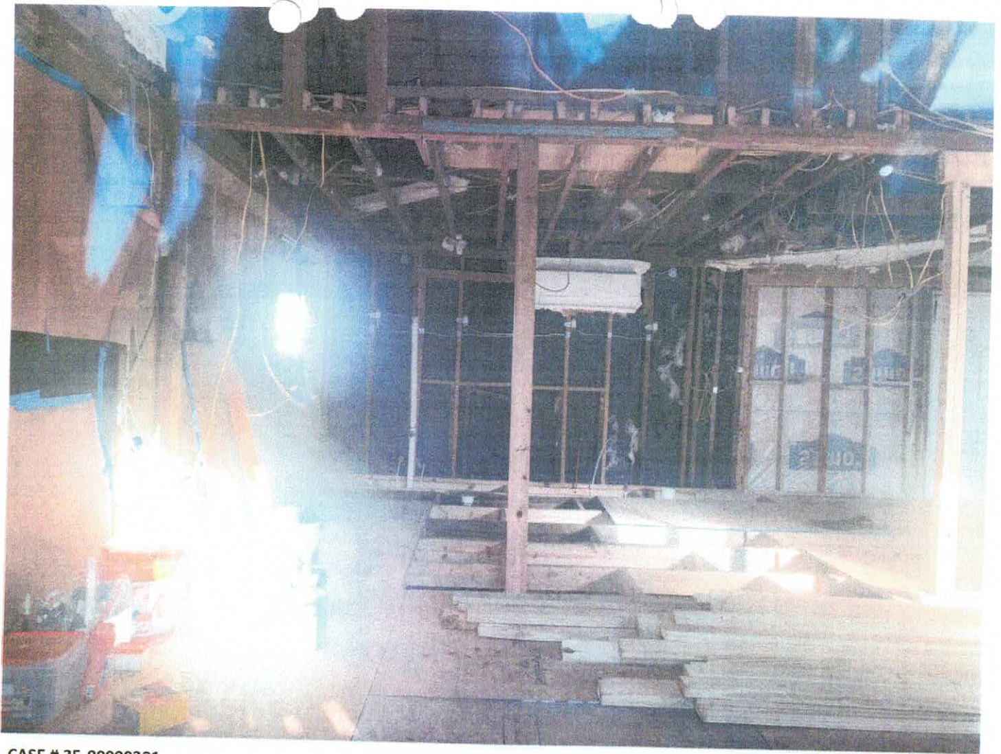
CASE # 25-80000391 SITE: 607 ISLAND DR INITIAL INSPECTION 1/10/2025 BY CEO MROLLESTON
