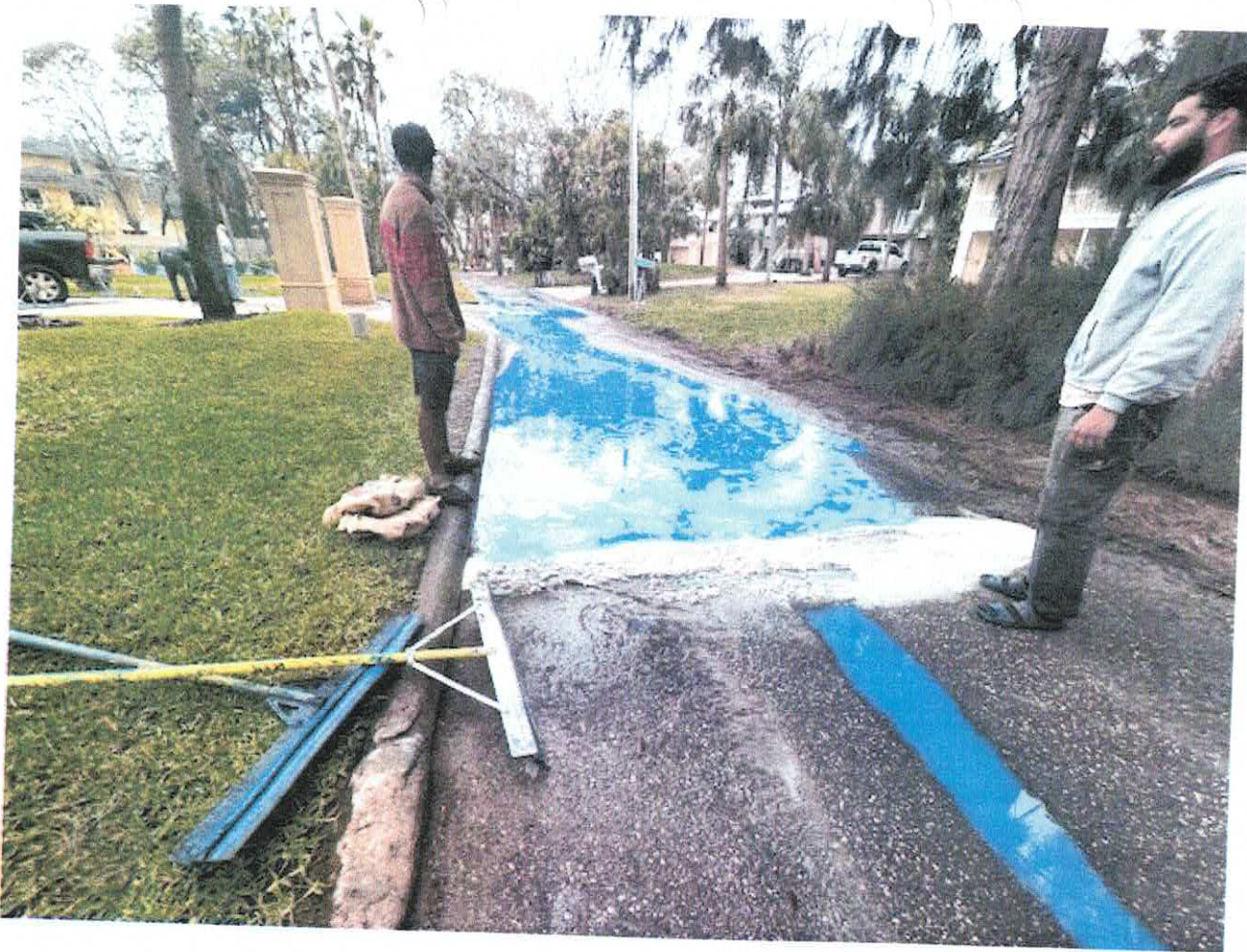
CASE 25-80000428 SITE: 1403 CIRCLE DR INITIAL INSPECTION 2/20/2025 STORMWATER - PAUL HOPKINS
