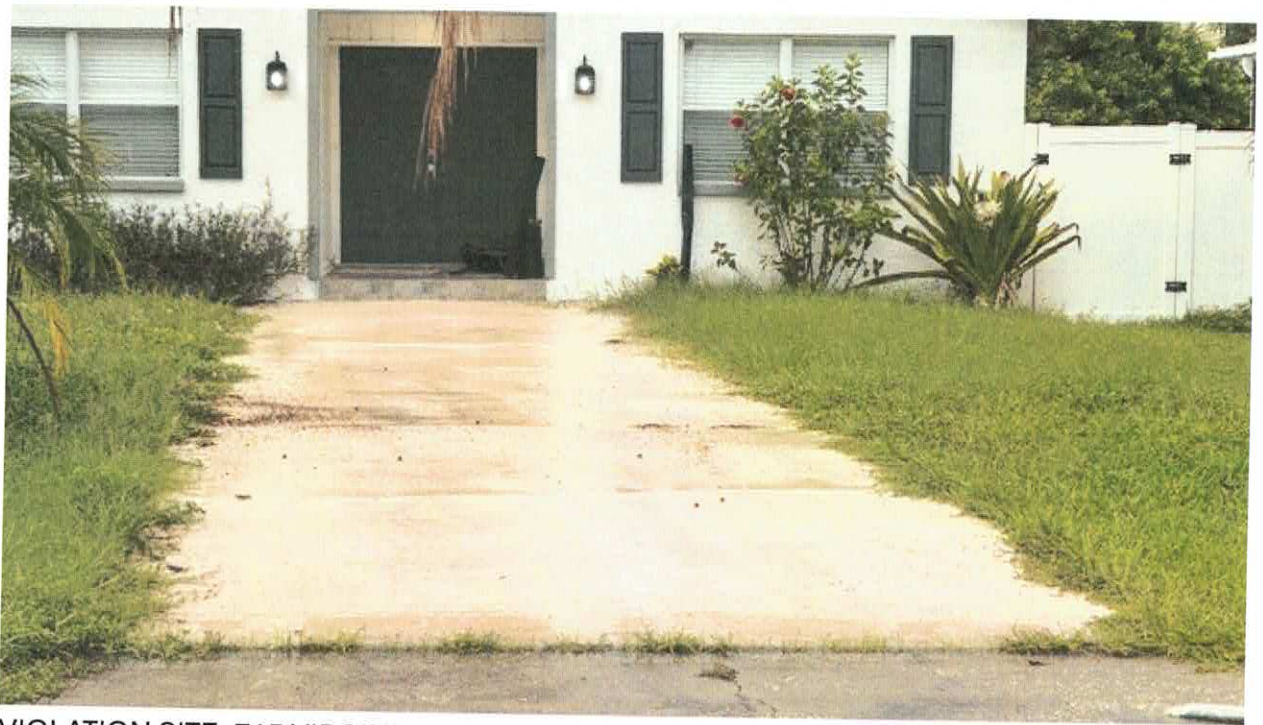
VIOLATION SITE: 715 VIRGINIA AVE, TARPON SPRINGS, FL 34689 Code Enforcement Supervisor: Anthony Boone Re-inspection 8/3/2026
