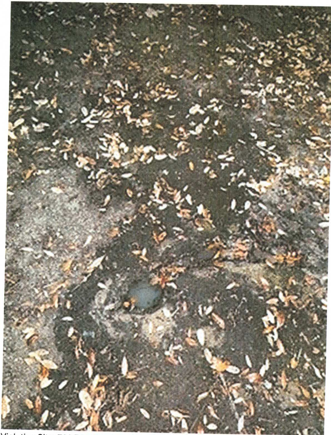
Violation Site: 706 E Tarpon Ave. , Tarpon Springs, FL 34689 Code Enforcement Officer: Michael Rolleston Initial Inspection 3/31/2026
