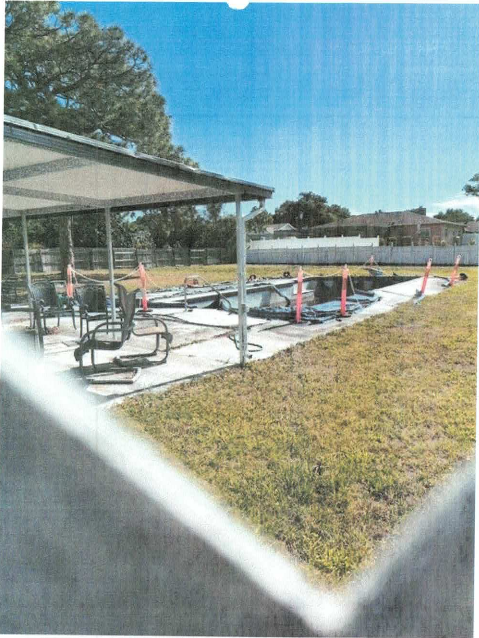
VIOLATION SITE: 1019 S FLORIDA AVE TARPON SPRINGS, FL 34689 INSPECTION 4/23/2026 BY CEO MICHAEL ROLLESTON
