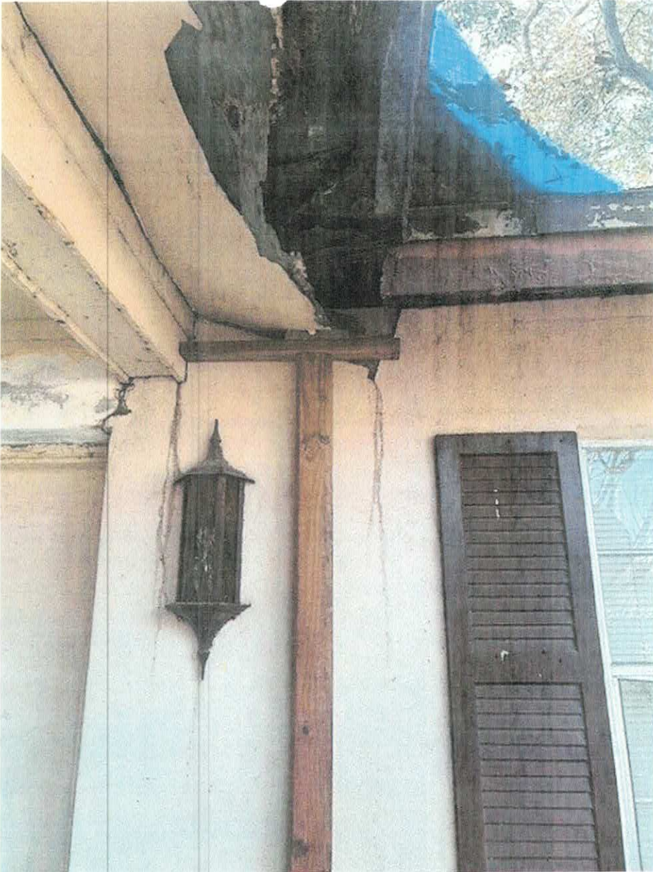
VIOLATION SITE: 1309 CROMWELL DR TARPON SPRINGS, FL 34689 INSPECTION 2/26/2026 BY CEO MICHAEL ROLLESTON
