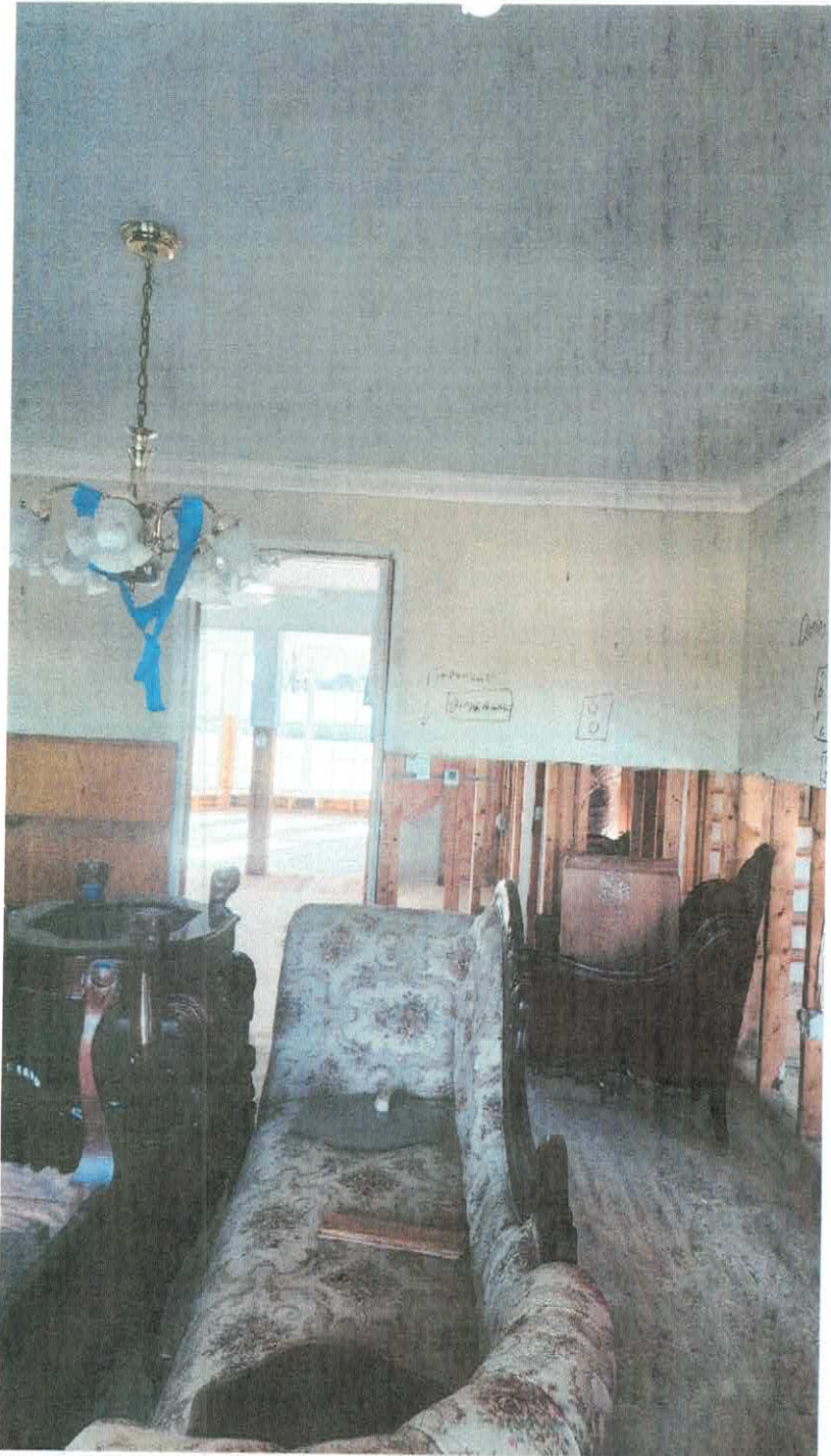
VIOLATION SITE: 1019 S FLORIDA AVE TARPON SPRINGS, FL 34689 INSPECTION 2/24/2026 BY CEO MICHAEL ROLLESTON
