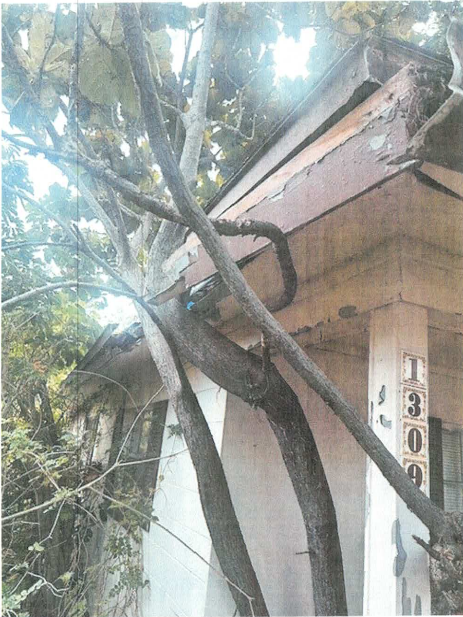
VIOLATION SITE: 1309 CROMWELL DR TARPON SPRINGS, FL 34689 INSPECTION 2/26/2026 BY CEO MICHAEL ROLLESTON
