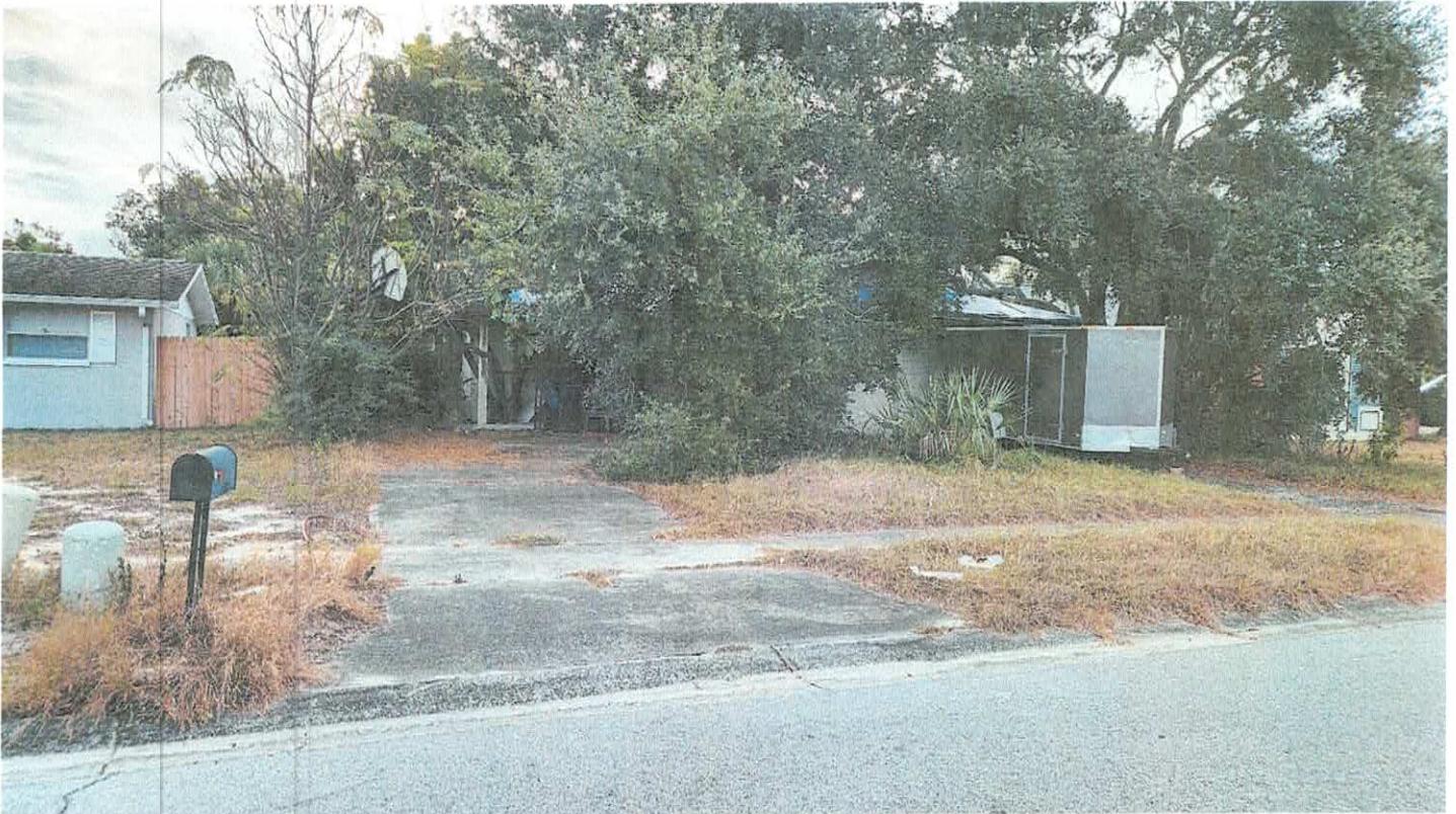
VIOLATION SITE: 1309 CROMWELL DR TARPON SPRINGS, FL 34689 INSPECTION 12/2/2026 BY CEO MICHAEL ROLLESTON
