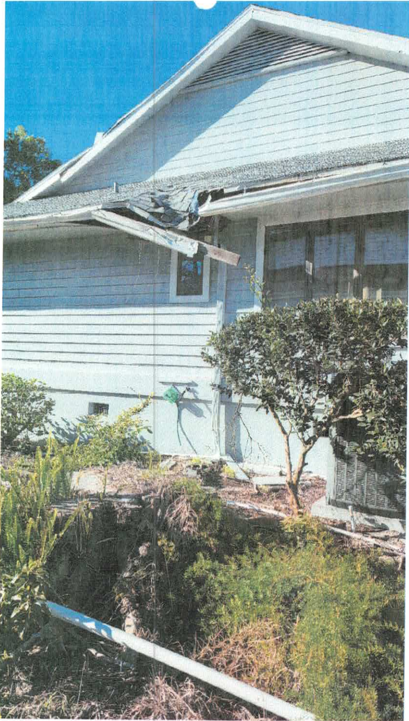
VIOLATION SITE: 1003 LAKE AVOCA DR TARPON SPRINGS, FL 34689 INITIAL INSPECTION 3/23/2026 BY CEO MICHAEL ROLLESTON
