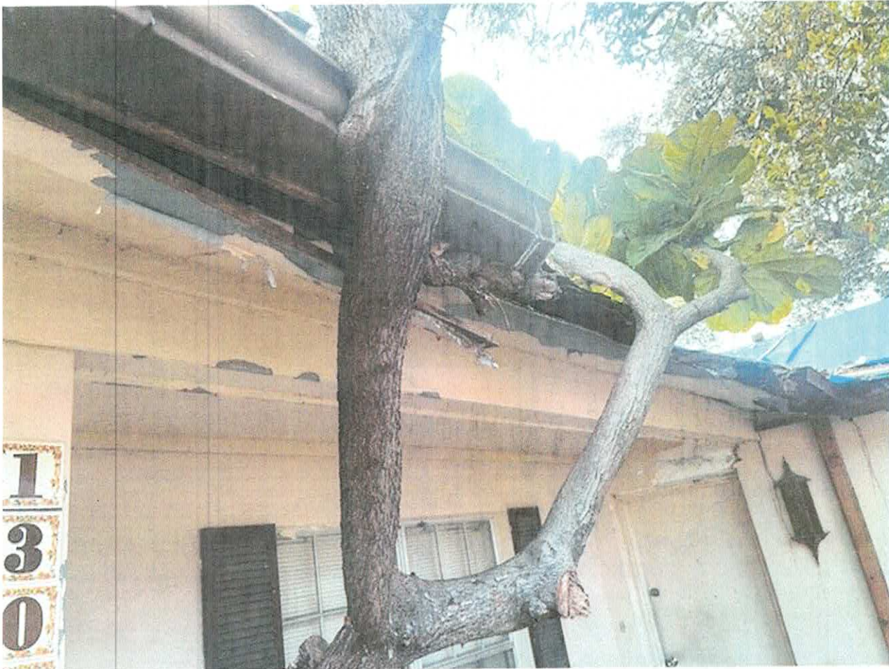
VIOLATION SITE: 1309 CROMWELL DR TARPON SPRINGS, FL 34689 INSPECTION 2/26/2026 BY CEO MICHAEL ROLLESTON
