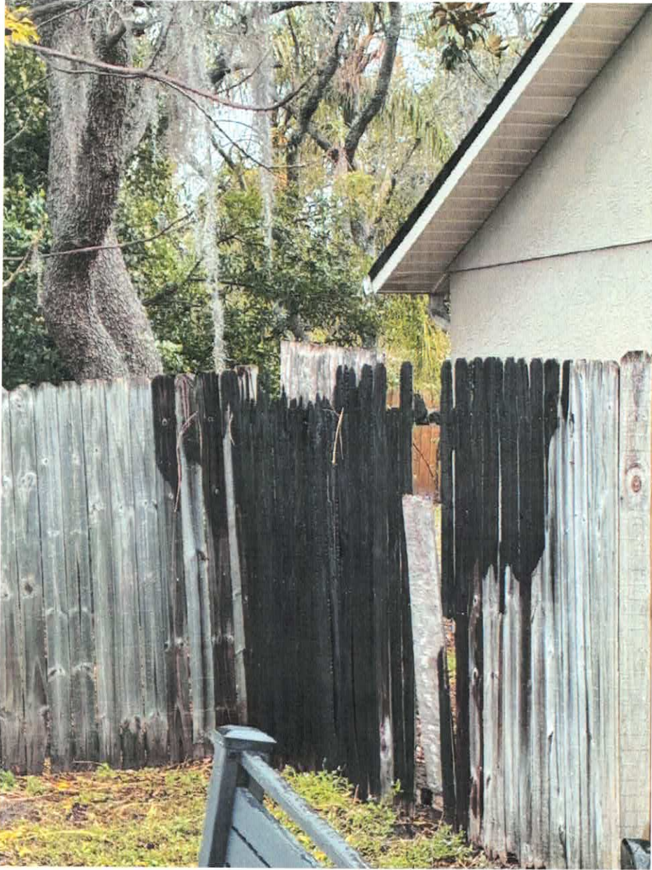
VIOLATION SITE: 1217 E LEMON ST TARPON SPRINGS, FL 34689 REINSPECTION 1/26/2025 CODE ENFORCEMENT OFFICER, MICHAEL ROLLERSTON
