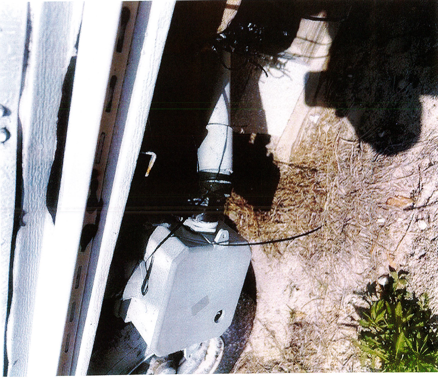
CASE # 24-80000323 VIOLATION SITE: LAKEVIEW DR TARPON SPRINGS, FL 34688 REINSPECTION 2/19/2026 BY CODE ENFORCEMENT SUPERVISOR ANTHONY BOONE
