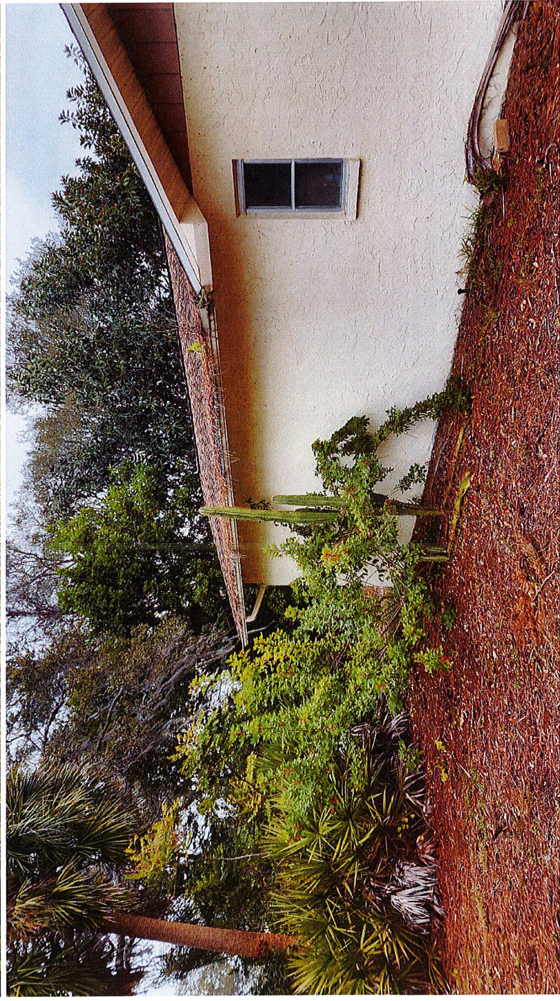
CASE # 26-80000758 VIOLATION SITE: 1508 POINSETTIA AVE TARPON SPRINGS, FL 34689 INSPECTION 2/5/2026 CODE ENFORCEMENT OFFICER MIKE ROLLESTON
