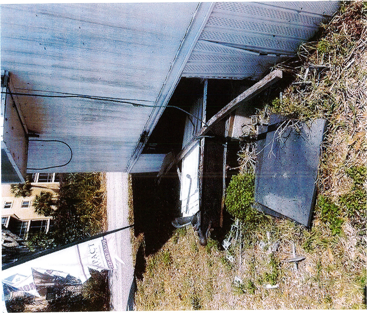
CASE # 24-80000323 VIOLATION SITE: LAKEVIEW DR TARPON SPRINGS, FL 34688 REINSPECTION 2/19/2026 BY CODE ENFORCEMENT SUPERVISOR ANTHONY BOONE
