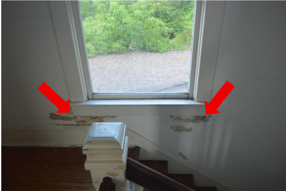
Photo 27: Damage at Sill of Window (Second Floor – West Side)
