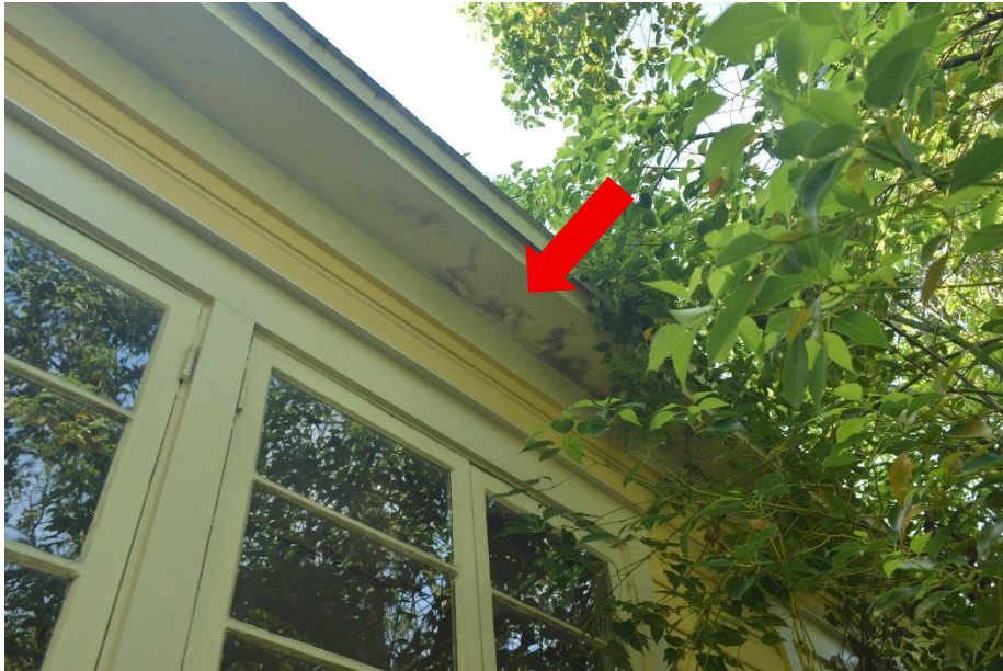
Photo 15: Water Staining at Soffit (West Elevation)
