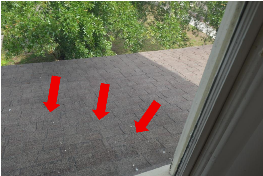
Photo 204: Granular Loss (Low Roof)
