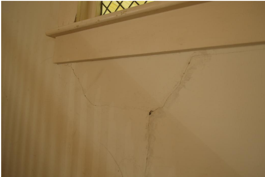
Photo 32: Cracked Wall Plaster (First Floor- West Side)
