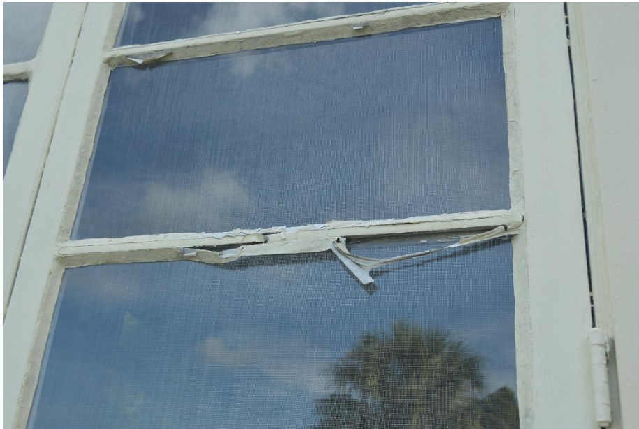
Photo 4: Broken Window Frame (South Elevation)
