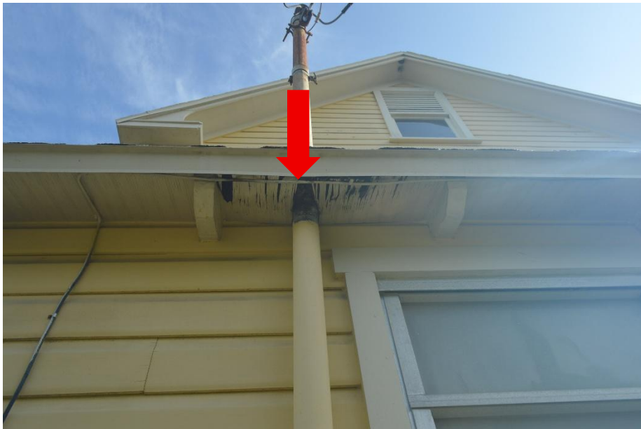
Photo 14: Damaged Soffit at Low Roof Penetration (South Elevation)
