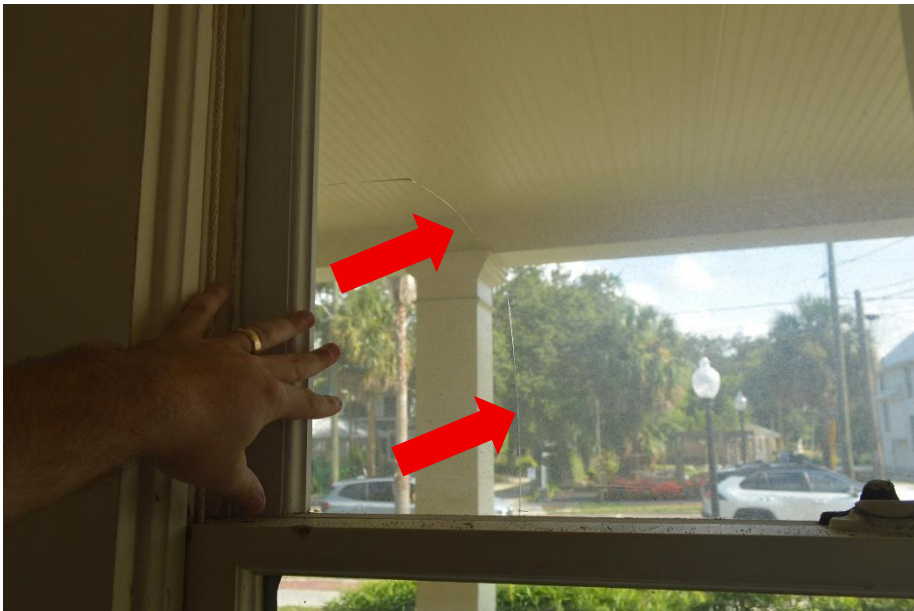
Photo 2: Broken Glazing (North Elevation)
