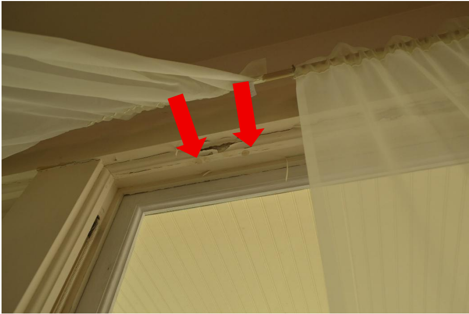
Photo 5: Water Staining at Window Below Low Roof (First Floor - North Elevation)
