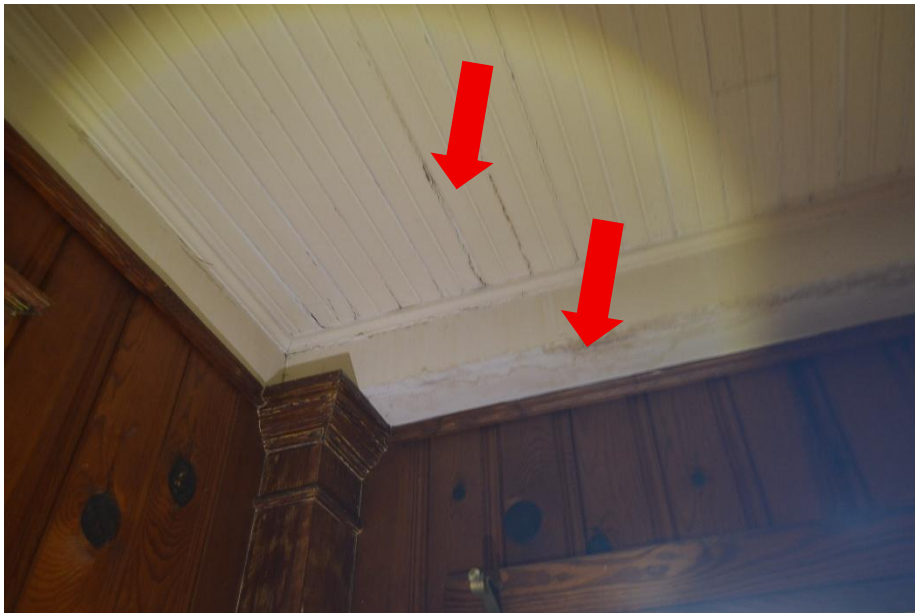
Photo 26: Ceiling Damage/Water Staining at Low Roof in Enclosed Patio
