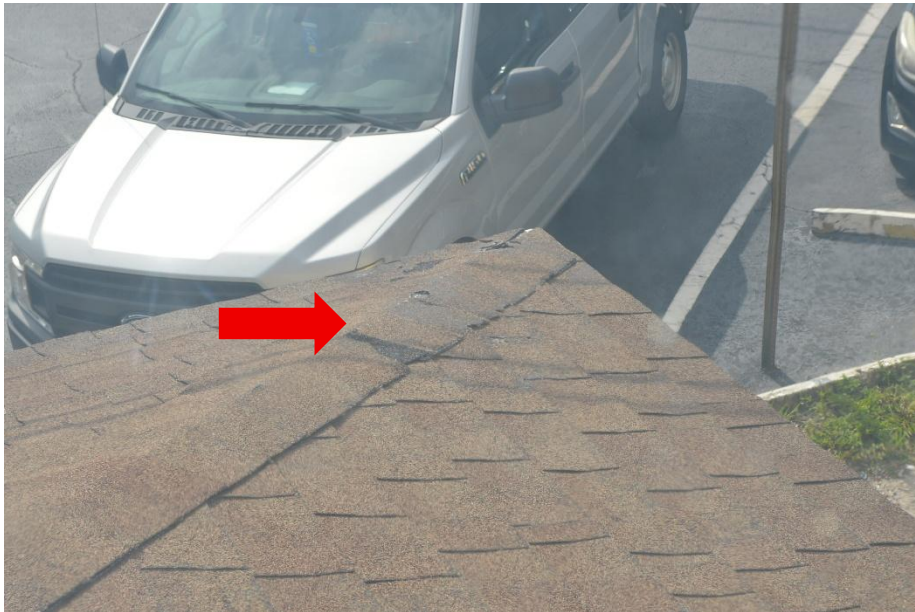
Photo 22: Torn/Damaged Hip Shingles (Low Roof)
