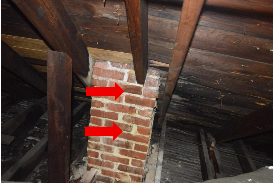
Photo 21: Water Staining to the South Chimney in the Attic
