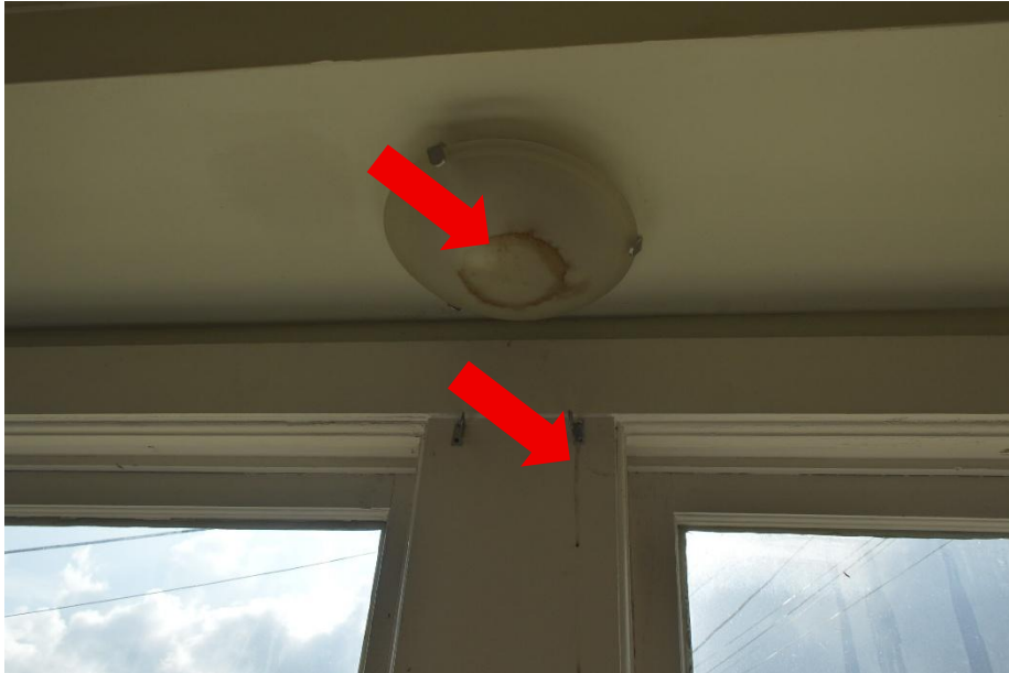
Photo 13: Water Staining at Light/Wall at East Wall (Kitchen)
