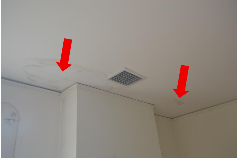
Photo 2921: Water Staining on Ceiling around North Chimney (Second Floor- Northeast)
