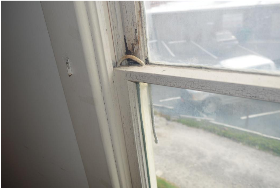
Photo 7: Inoperable Window (Second Floor - East Elevation)
