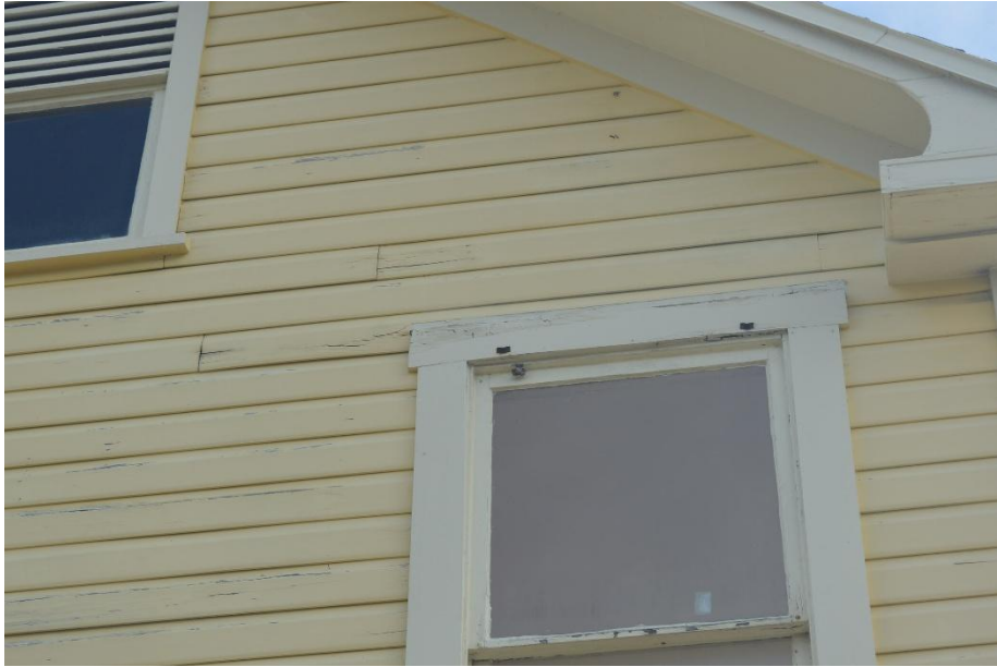
Photo 17: Deteriorated Exterior Paint (South Elevation)
