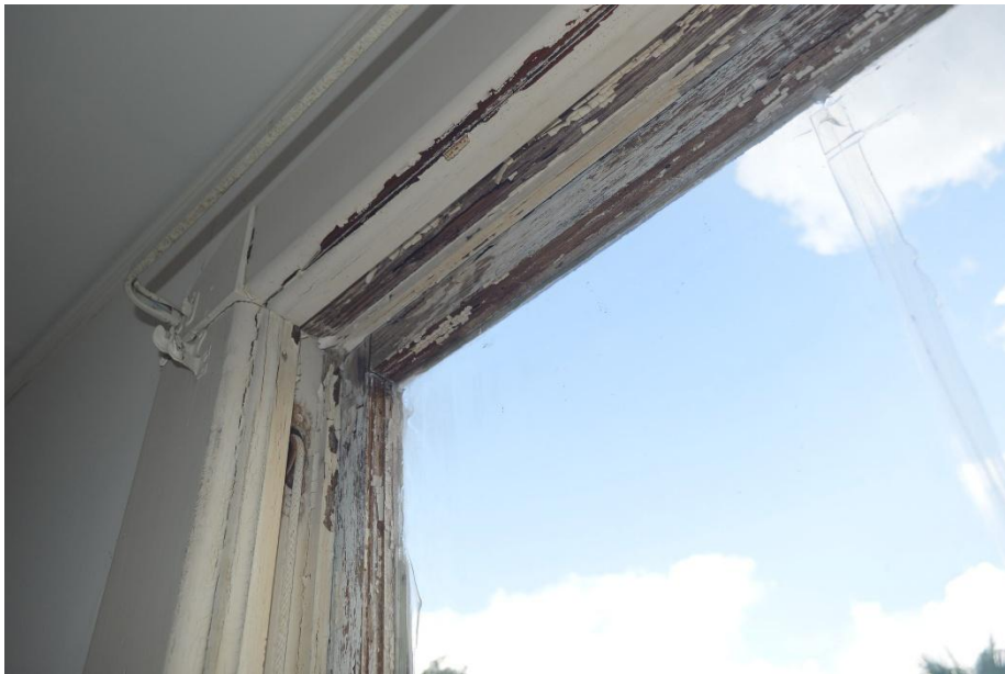
Photo 6: Damaged/Rotted Window Frame (Second Floor - North Elevation)
