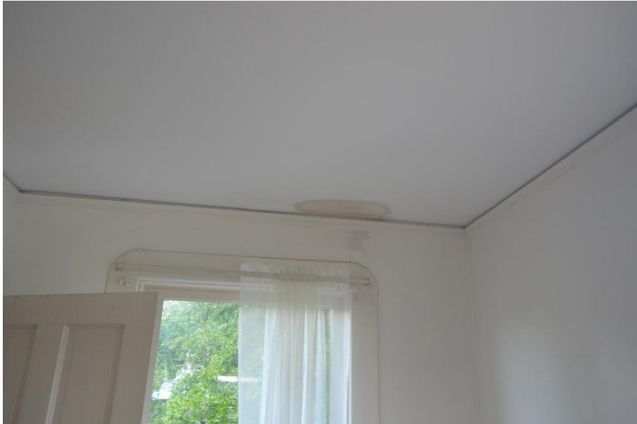
Photo 28: Ceiling Staining on Second Floor (Second Floor - Northwest)
