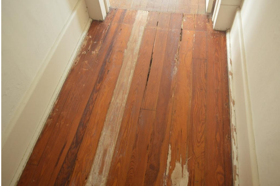
Photo 25: Wood-Boring Organism Damage to Wood Flooring (Second Floor)
