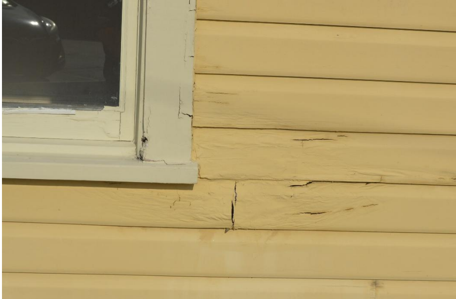
Photo 11: Damaged/Rotted Siding around Window/Opening (East Elevation)
