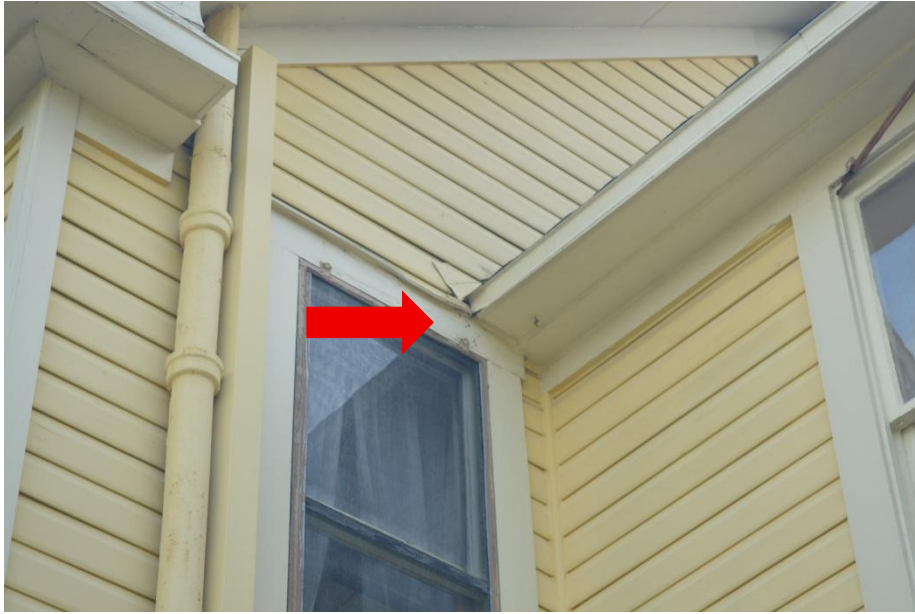
Photo 19: Water Damaged/Rotted Siding/Trim at High Roof to Wall Interface (West Elevation)
