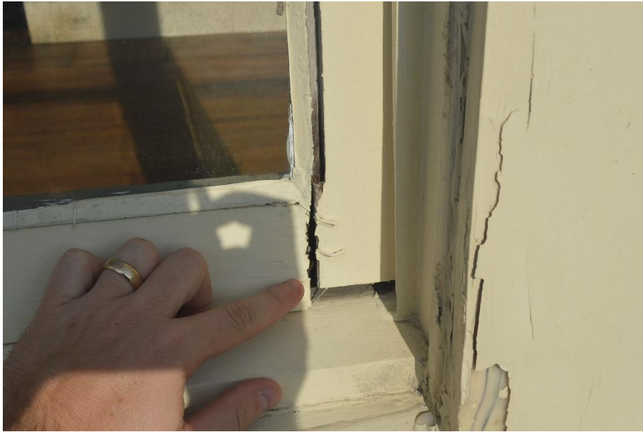
Photo 1: Broken Wood Window Sash (East Elevation)
