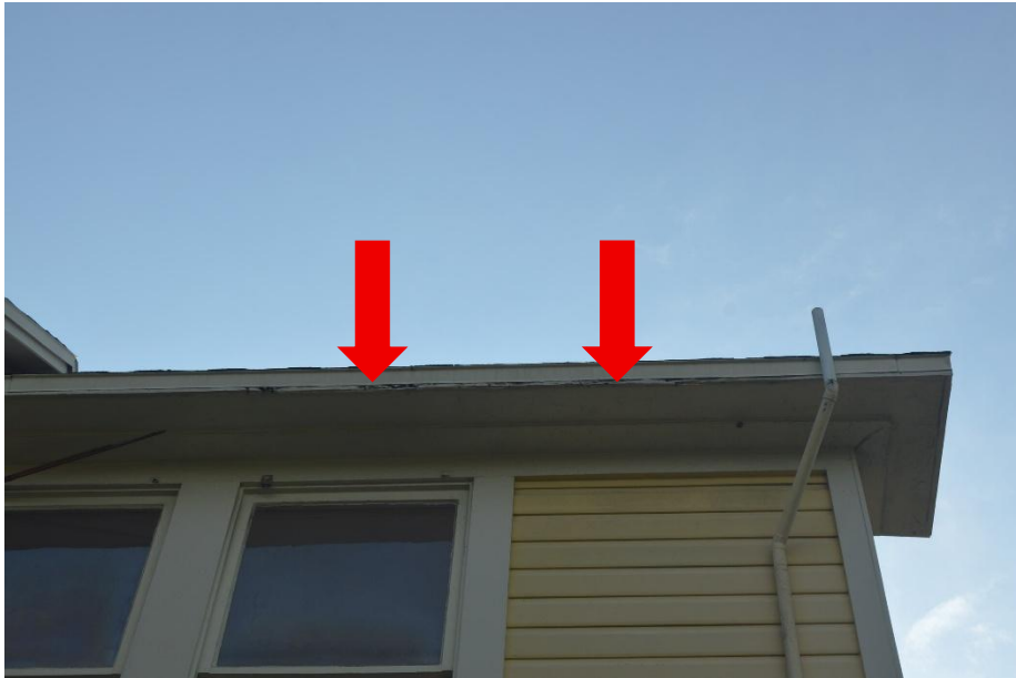
Photo 18: Rotted/Damaged Roof Fascia (West Elevation)
