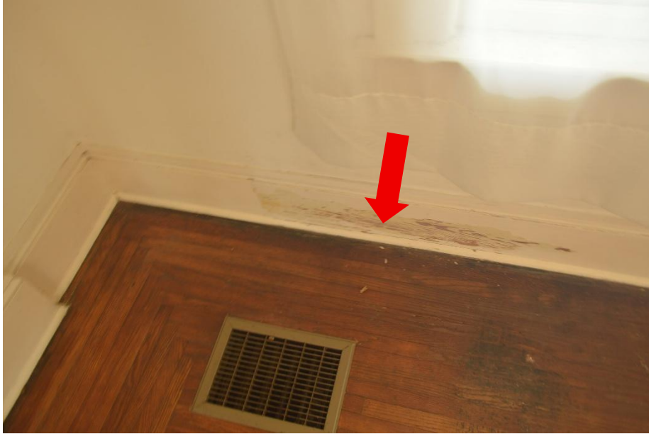
Photo 35: Deteriorated Paint (Kitchen)
