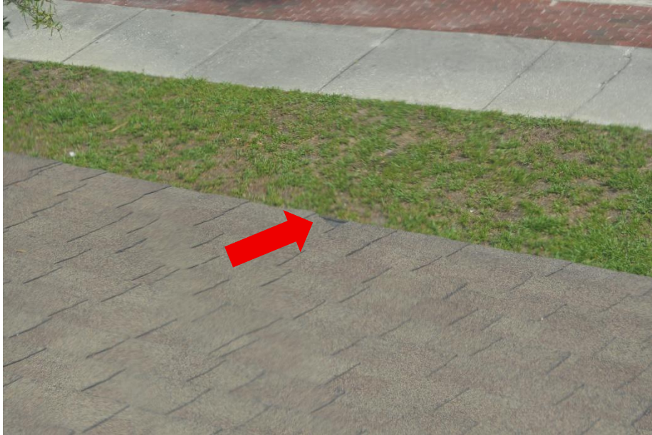
Photo 193: Torn/Damaged Shingles (Low Roof)
