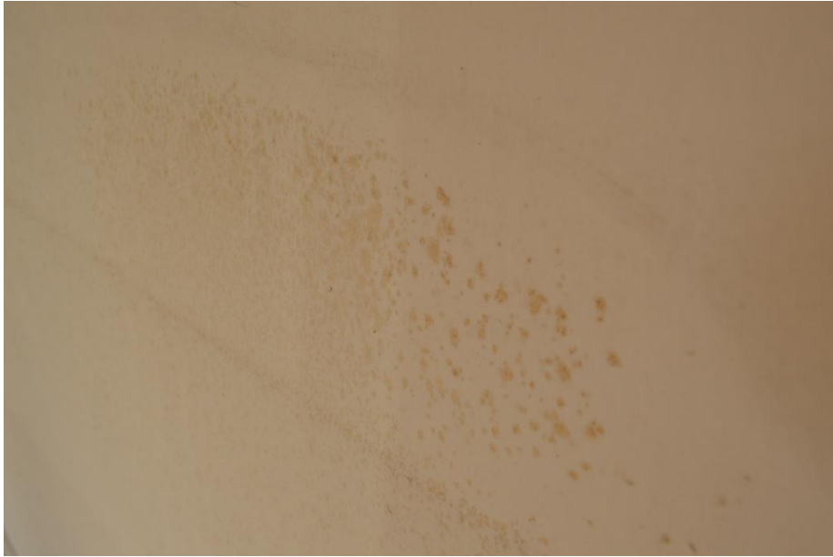
Photo 33: Possible Mold Presence (First Story – Middle Room)
