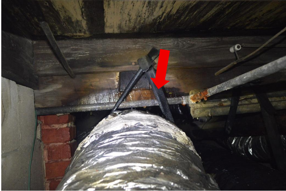
Photo 37: Active Water Leaking in Crawlspace
