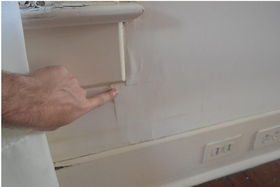
Photo 30: Water Damage under Window (Second Floor – North Side)
