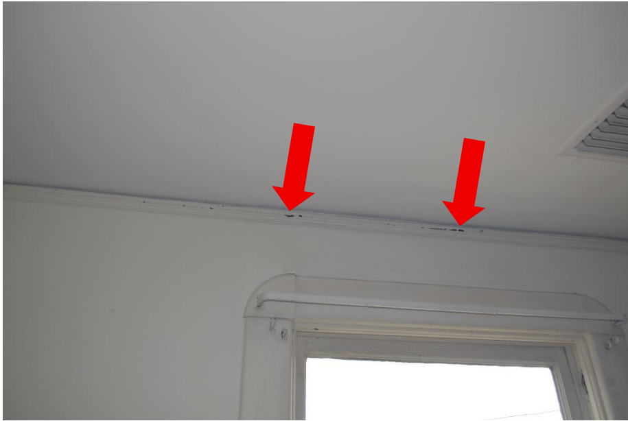
Photo 31: Wood Boring Damage to Interior Wood Trim (Second Floor- East Side)
