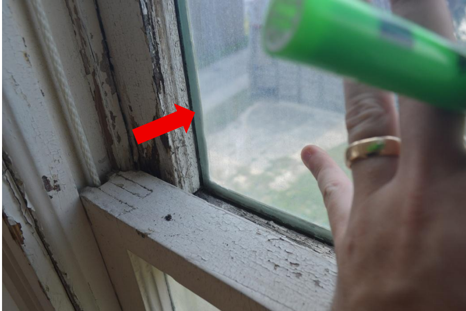
Photo 3: Failed Window Repair (Sealant at Glazing-South Elevation)
