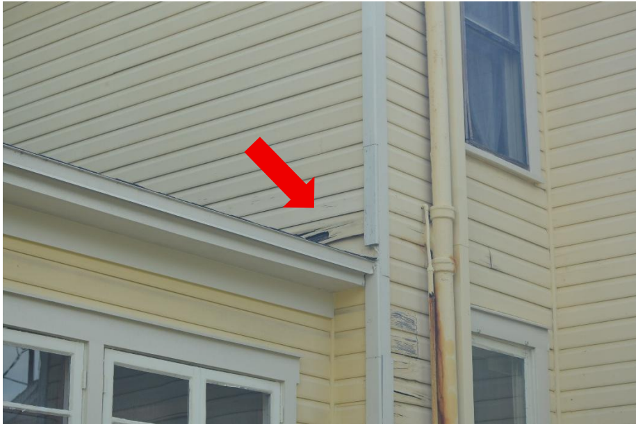
Photo 20: Water Damaged/Rotted Siding/Trim at Low Roof to Wall Interface (West Elevation)
