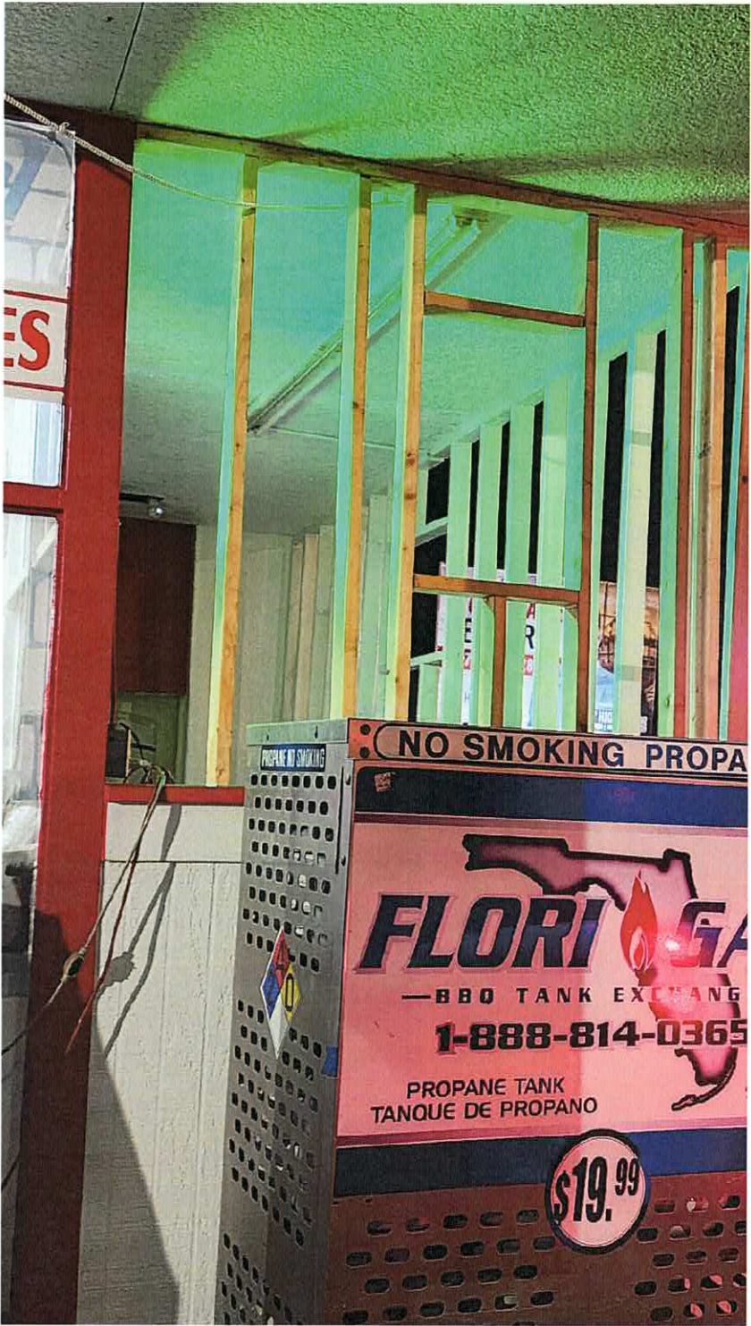
VIOLATION SITE: 4 S PINELLAS AVE TARPON SPRINGS, FL 34689 INITIAL INSPECTION 12/12/2025 CEO MR
