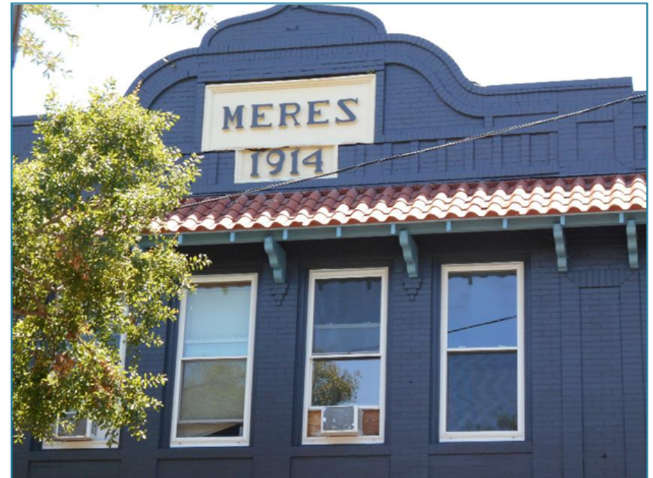
Figure 126: Replacement windows on the second floor of the Meres Building match the historic window openings and type but not material.
